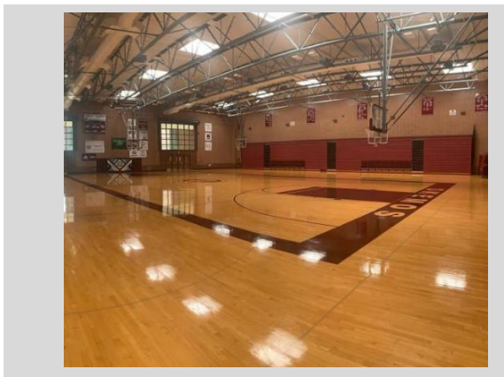
LED Lighting at High School Gymnasium
